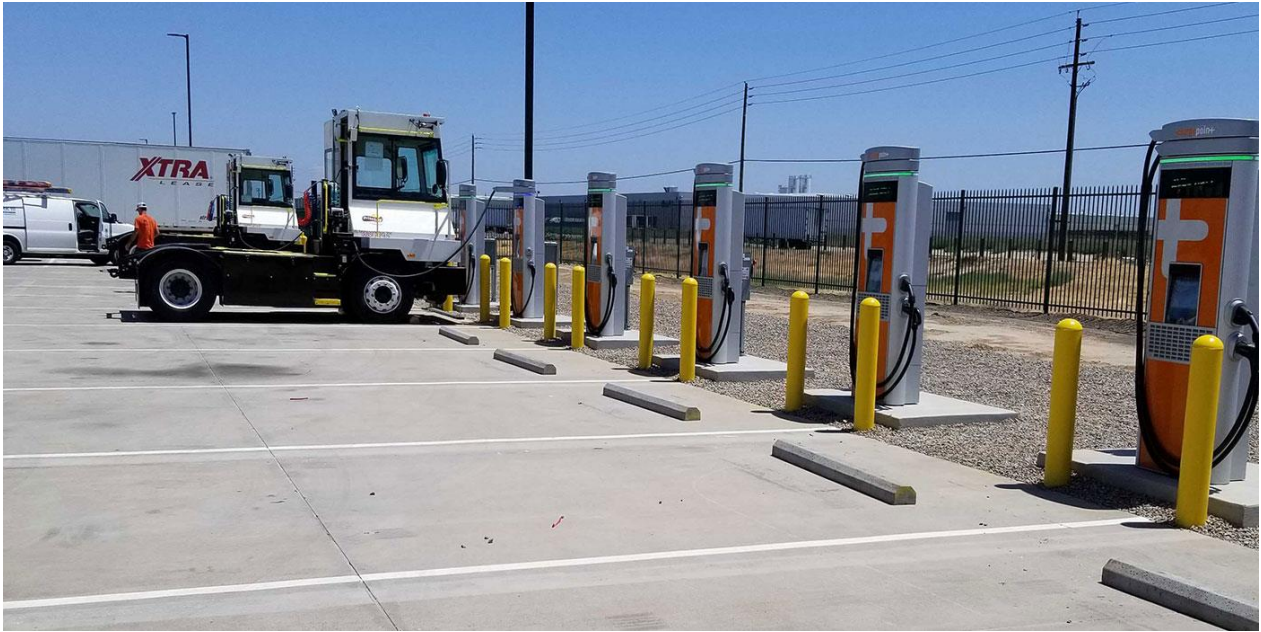
Figure 5-29 Snapshot of Electric Freight Vehicle Depot Charging Facility
